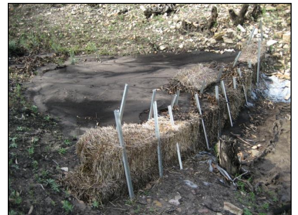
Figure 4: Overflowing sediment barrier trap
